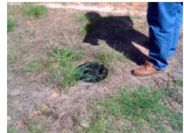
Uncapped water meter—have utility replace cover or make one
