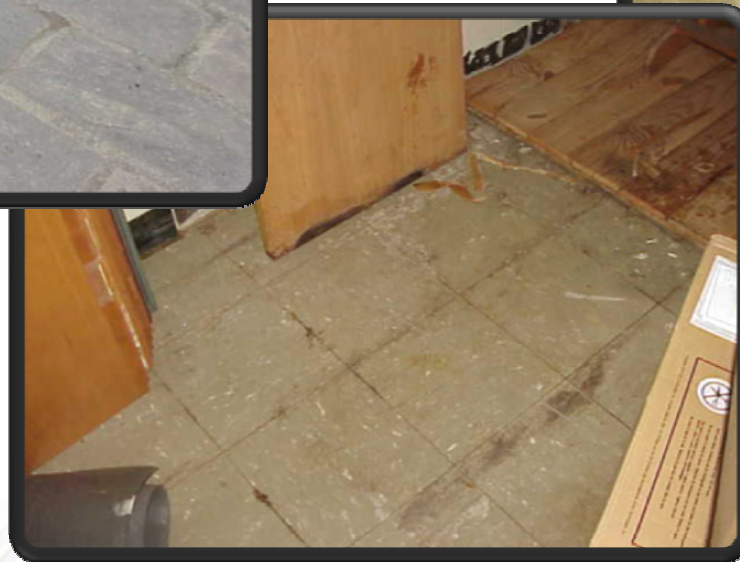
Damaged Flooring and Walls
