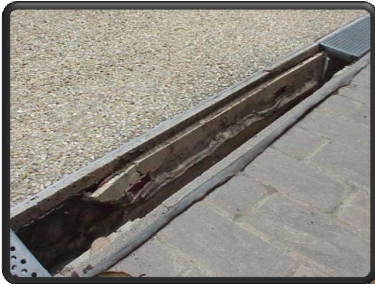
Storm Drains in Disrepair
